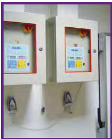
Controllo temperatura in celle frigo
